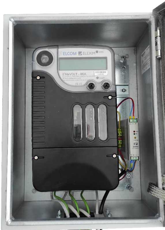
Figure 12 Real installation of device E 2 MeVOLT
